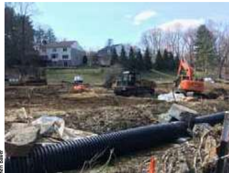
THE ENTIRE FALLSREACH STREAM, A TRIBUTARY OF WATTS BRANCH (WEST OF I-270) IS RUNNING THROUGH THE BLACK PIPE DURING CONSTRUCTION (3/19/2019).
