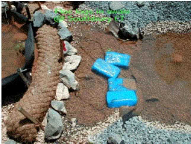
Figure 8 - Reduce Turbidity using Floc Logs
